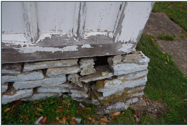
Figure 17: Collapse and cracking at southwest corner
