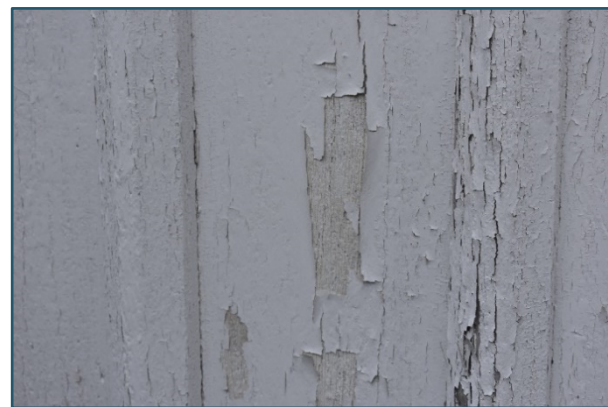
Figure 40: Layers of peeling paint
