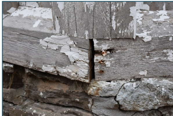
Figure 35: Separating at beam joint above foundation
