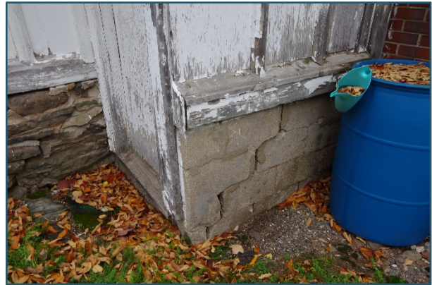
Figure 7: Moisture draining towards foundation near shed
