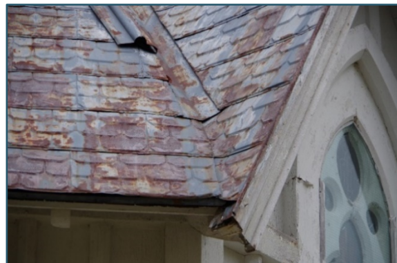
Figure 20: Missing flashing at roof valley
