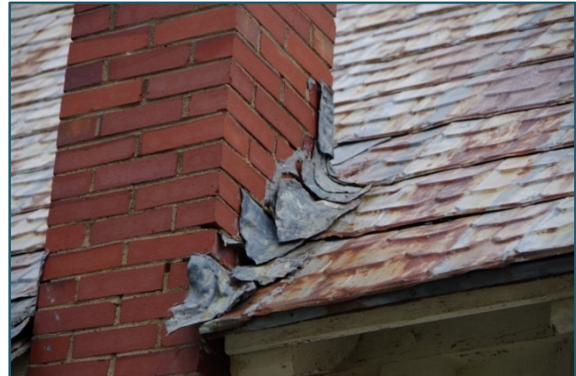
Figure 48: Failed chimney flashing
