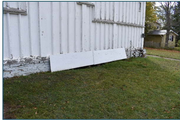
Figure 18: Boarded up collapsed west foundation
