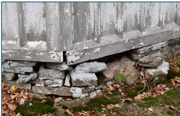
Figure 13: Collapse below northeast apse corner, note separation at sill beam joint
