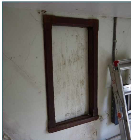
Figure 47: Boarded up narthex window
