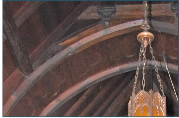
Figure 29: New cord near top of arch
