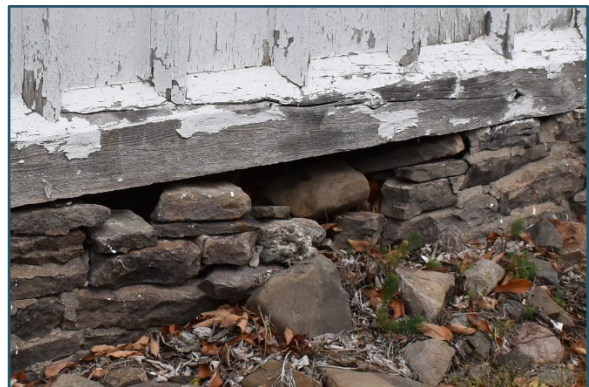
Figure 14: Partial collapse in south wall near southeast corner, note checking in sill beam
