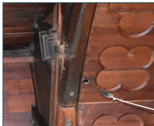
Figure 27: Detached bell tower post at arch peak
