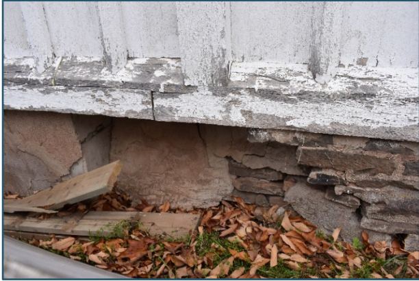
Figure 15: Parging failure and collapse at block wall near chimney
