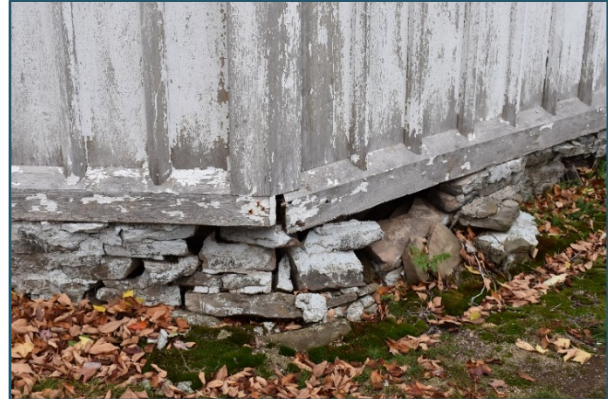
Figure 38: Cracked foundation and separated sill beams at northeast corner
