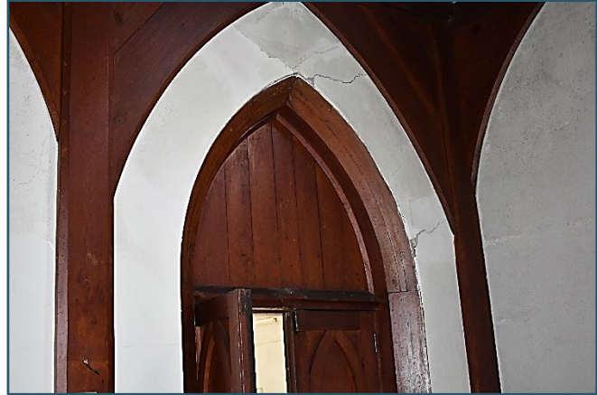
Figure 43: Crack above door arch
