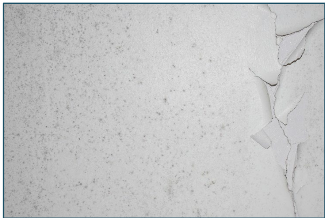
Figure 44: Mildew on west wall
