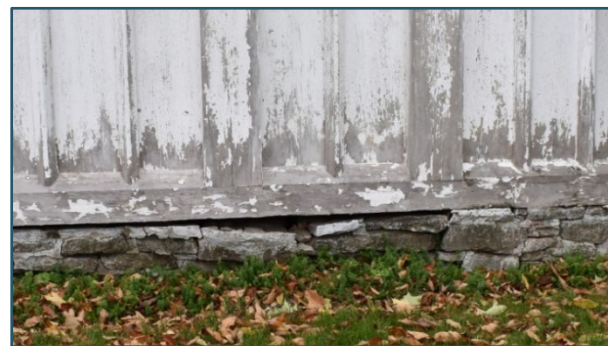
Figure 39: Failed foundation beneath chancel arch
