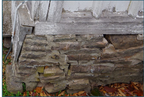
Figure 16: Diagonal cracking and inappropriate plywood repair at southeast narthex corner
