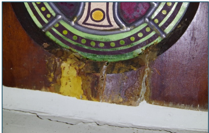
Figure 52: Cracked stained glass window frame
