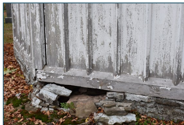
Figure 37: Gap at northeast corner
