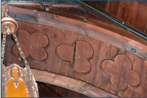
Figure 28: Cracks and triangular gaps in north arch panels.
