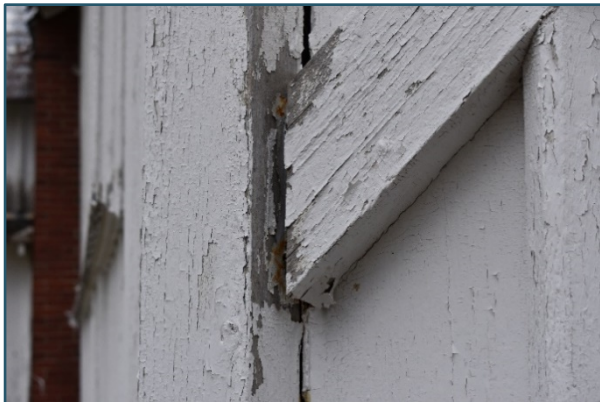
Figure 34: Separating joint at post
