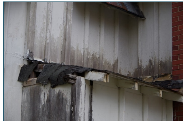
Figure 49: Deteriorated shed roof and water damage on wall
