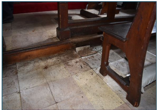
Figure 31: Warped tiles near chancel porch.
