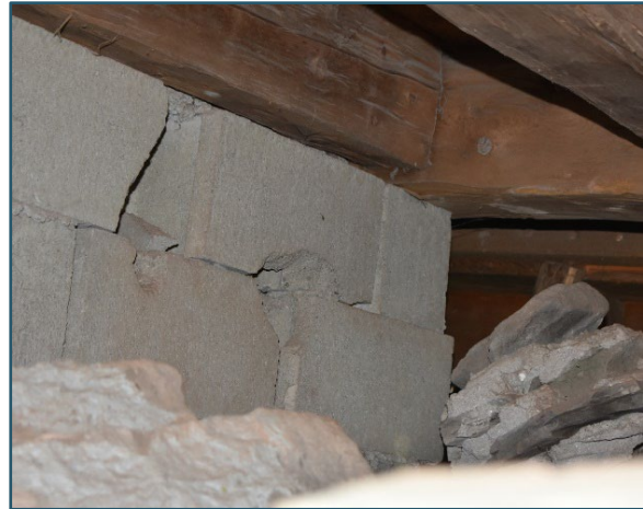
Figure 9: Damaged concrete block wall
