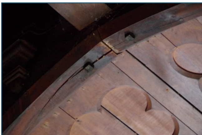
Figure 26: Arch joint separating and splitting at connection
