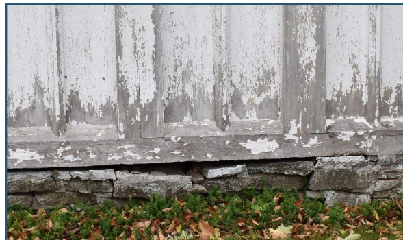
Figure 12: Partial collapse below small north window
